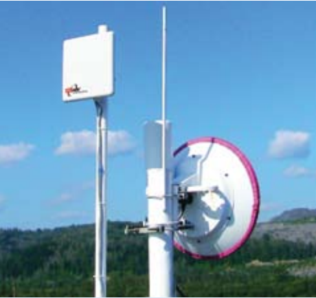
Gas utility connectivity, Siberia
