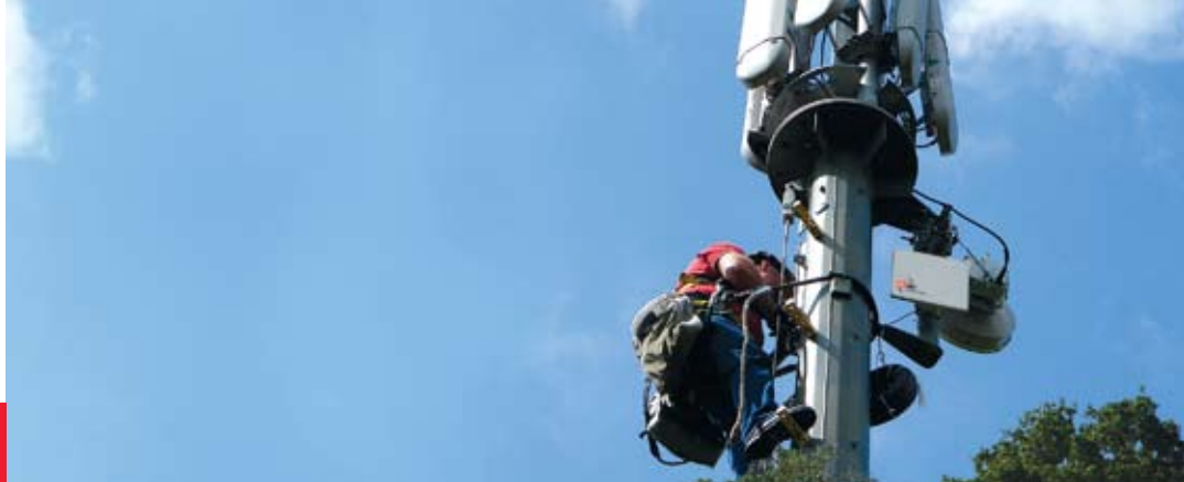
Cellular backhaul installation, USA
